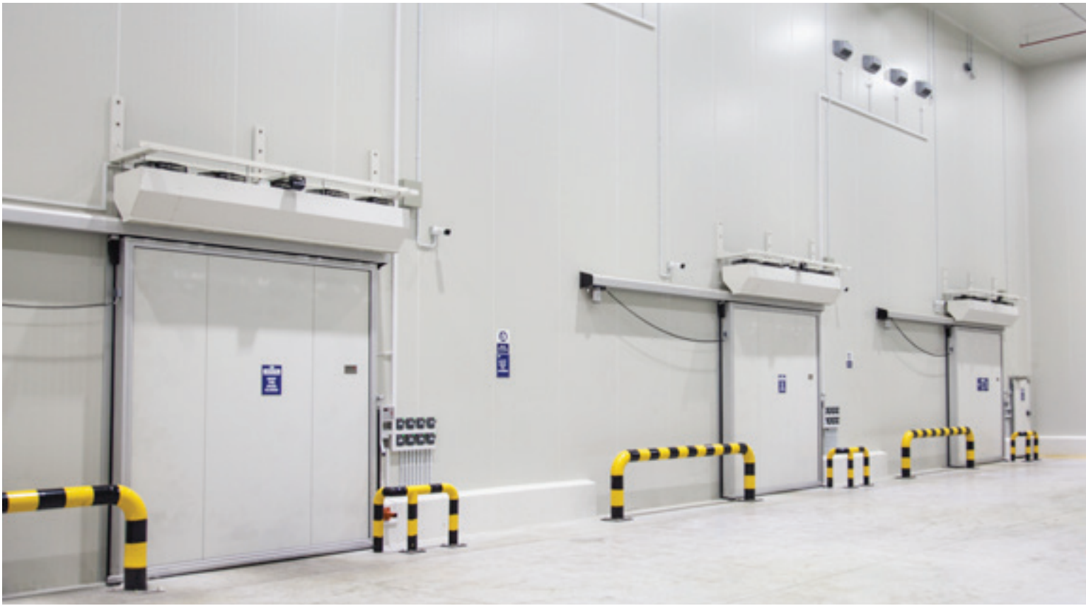
COLD STORE SLIDING DOORS (CHILLER & FREEZER)
