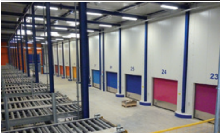
AIR LOCK DOORS
