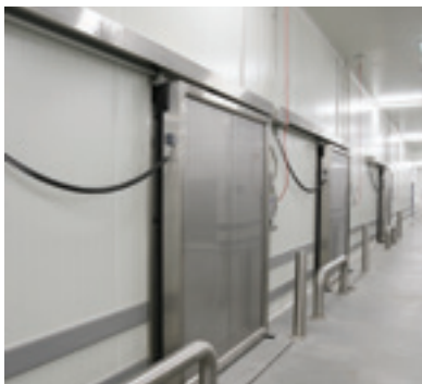
Electrically Operated Doors
