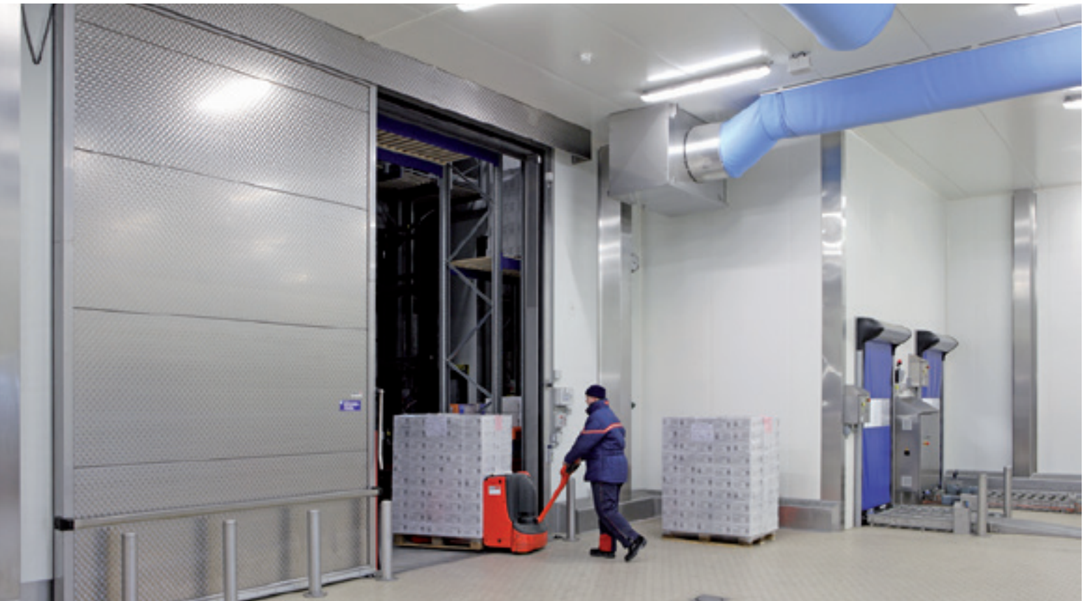
STAINLESS STEEL DOORS (CHILLER & FREEZER)
