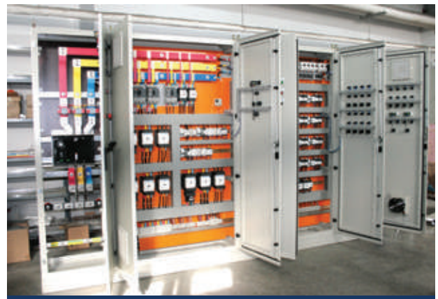
SWITCHGEAR AND CONTROL PANELS
